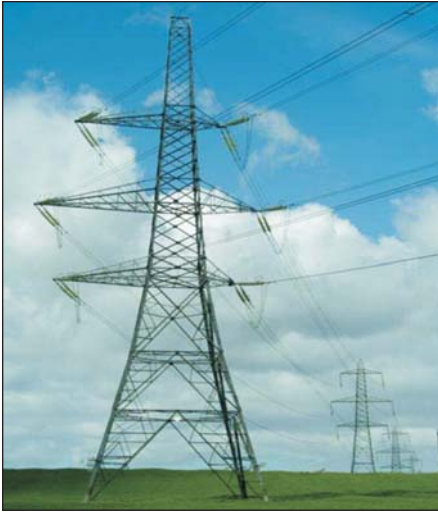
Figure 2 · Electric power line.
