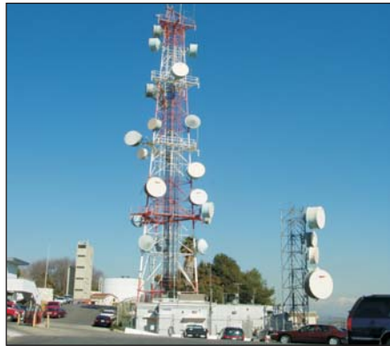
Figure 4 · Microwave communication site.
